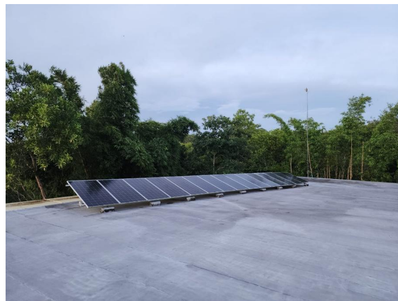
Figure 6. Existing Solar Panel Infrastructure Under Evaluation for RO Plant Integration
